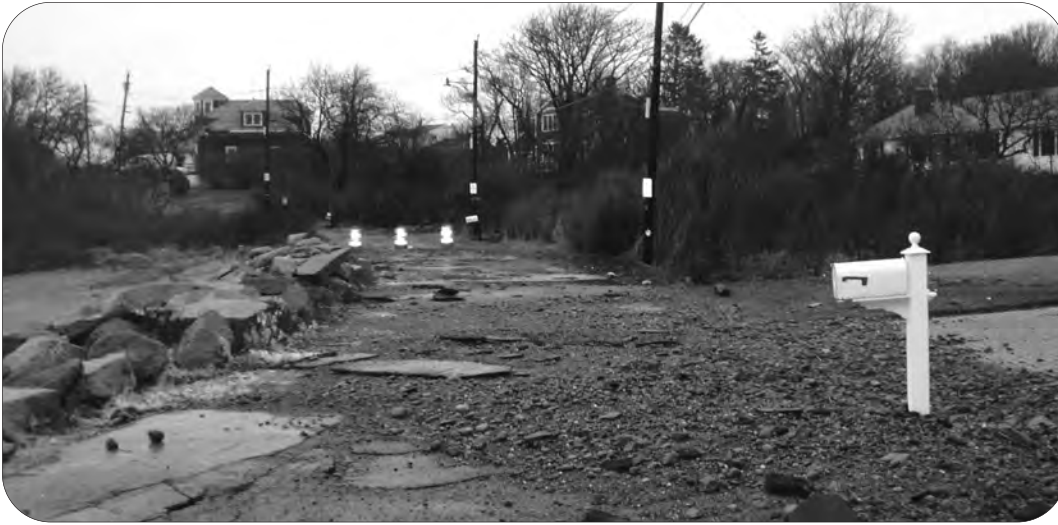
In addition to being costly to repair, roads damaged by storms can become hazards for rescue personnel and others. This road in Rockport, Massachusetts, was destroyed by a 2007 nor'easter.
